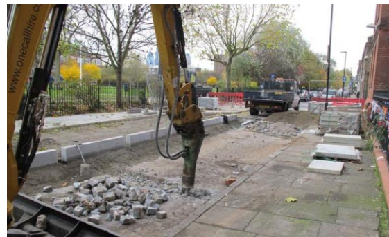
Figure 2 Re-levelling road bed, Derbyshire Street pocket park, Bethnal Green, London (courtesy of London Borough of Tower Hamlets)
