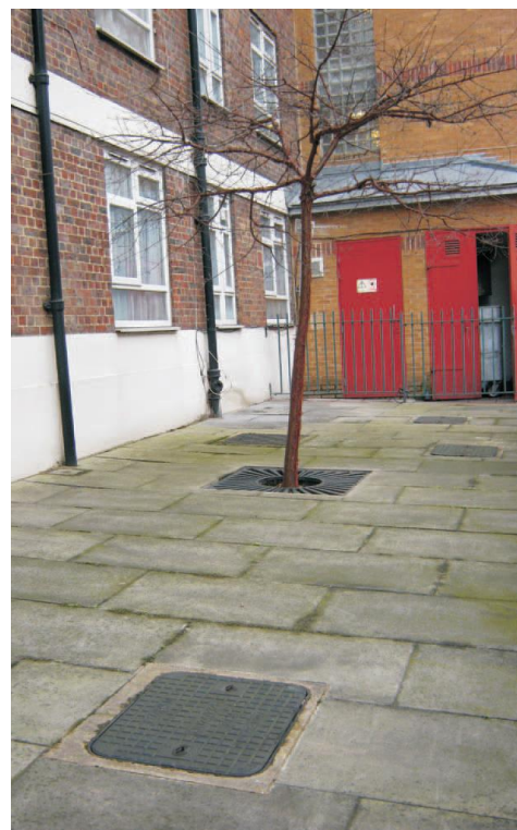
Figure 4 Part of the Kingsmead estate before retrofitting a rain garden took place
