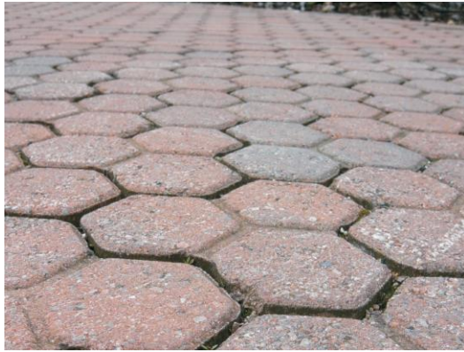
Figure 1 Permeable paving on a high density development in Stamford
