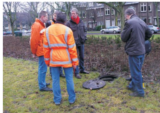
Figure 2 Workers standing on top of a shallow subterranean infiltration tank at a housing area in The Hague, Holland
