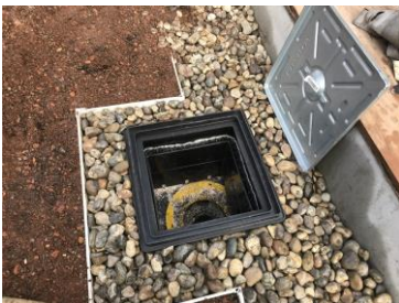
Blue roof restrictor chamber
