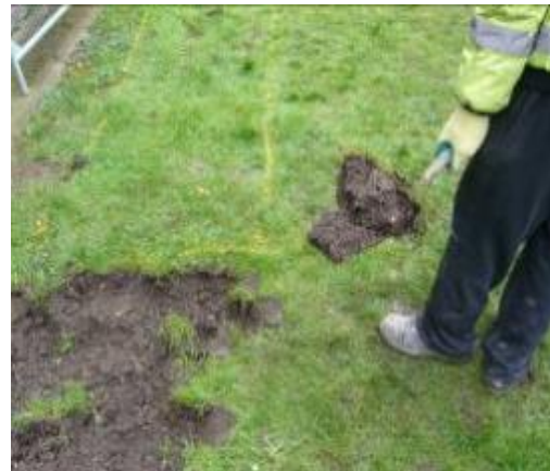
Figure 6 Ground breaking. All turf and soil was retained on site to be incorporated into the final design
