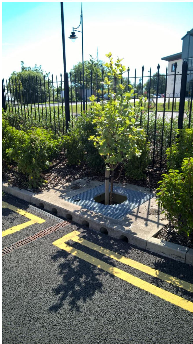
Fig 1: Biofilter unit with combined kerb inlet and channel drain inlet
