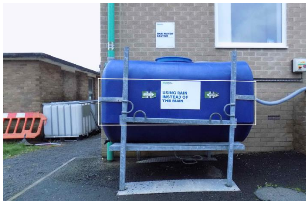
Figure 3 Rainwater harvesting tank at Cramlington Treatment Works
