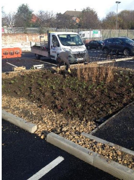
Fig 2 Rain garden at Howdon Treatment Works
