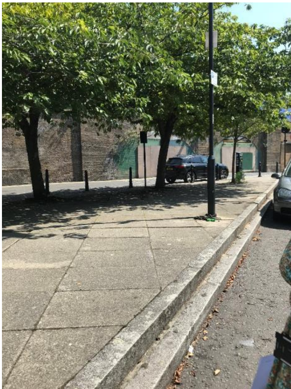
Figure 3: Level difference between island and adjacent carriageway
