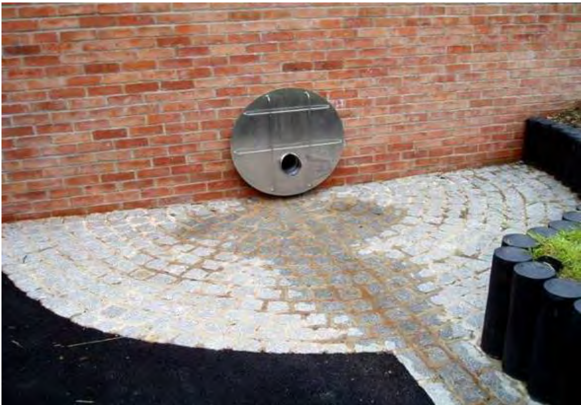
Figure 2: The stainless steel spout feature and sett apron leading to a sett channel
