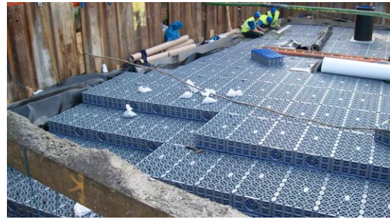
Figure 9 Retrofitting geo-cellular storage as part of a wider scheme with storage swale in a grass verge to reduce the risk of flooding from the surface water system.
