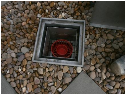
Restrictor Chamber & RWO Level 60
