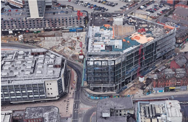
Installation of the blue roof attenuation system and insulation boards on main roof Level 60
